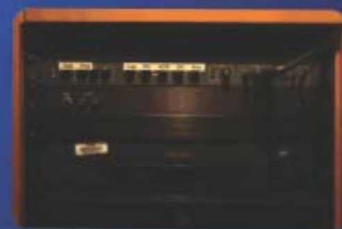
Lower Control Panel
